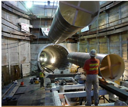
Service Pipe Entering the Tunnel
