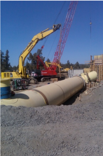
108" Penstock Pipe Entering the Powerhouse
